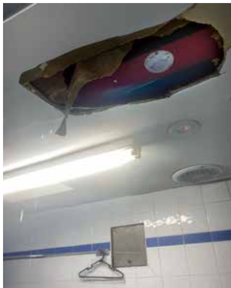
RAIN POURING PAST WIRING THROUGH DAMAGED ROOF
