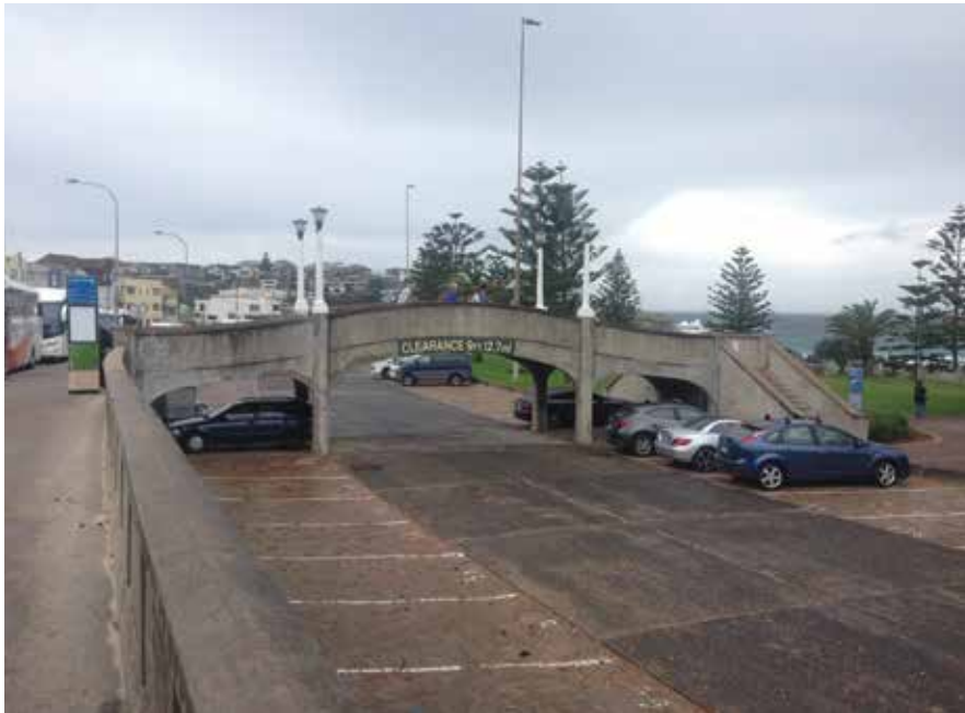
PEDESTRIAN BRIDGE SOUTH OF CAMPBELL PARADE, NORTH OF BONDI PAVILLION AND ARCHER PARK, VIEWED FROM CAMPBELL PARADE JUST NORTHWEST OF THE BRIDGE / PHOTO CREDIT PHILIP MALLIS
